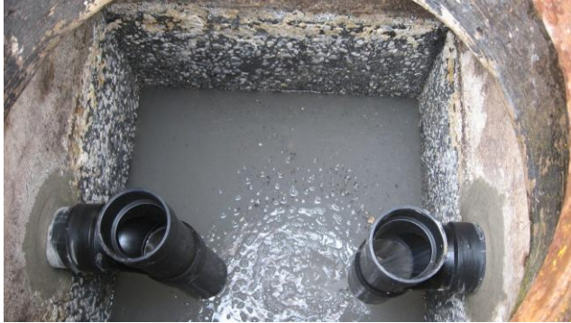
A well-cleaned and compliant grease interceptor.
