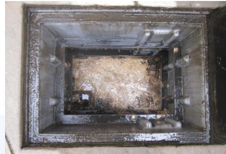
Interceptor operating correctly.
