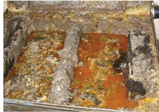
Interceptor pumped out - NOT cleaned to standards.
